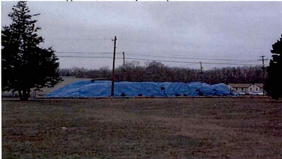
ID-27 soil pile storage area near the excavation site. The area is covered top and bottom by poly tarps and is bordered by hay-bails to control any soil runoff as a precaution. Approx. 4,000 cubic yards of soil were removed.
