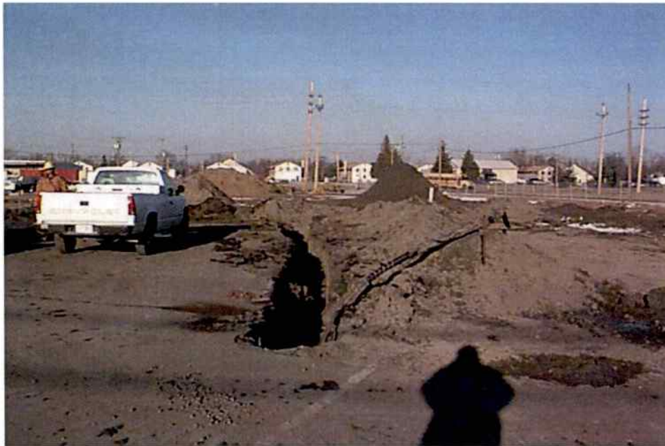
Jan 14, gas pipe excavation from the fuel distribution/railroad track area facing north. This pipe led us to the most contaminated area (the rail-car off-loading area) which is believed to be the source area for the fuel contamination.
