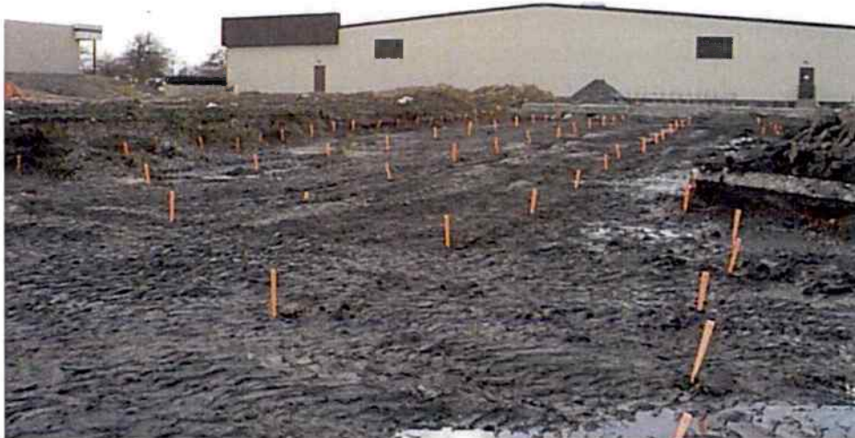
West excavation area (railroad track area) sample results show a clean excavation and the area is being backfilled.
