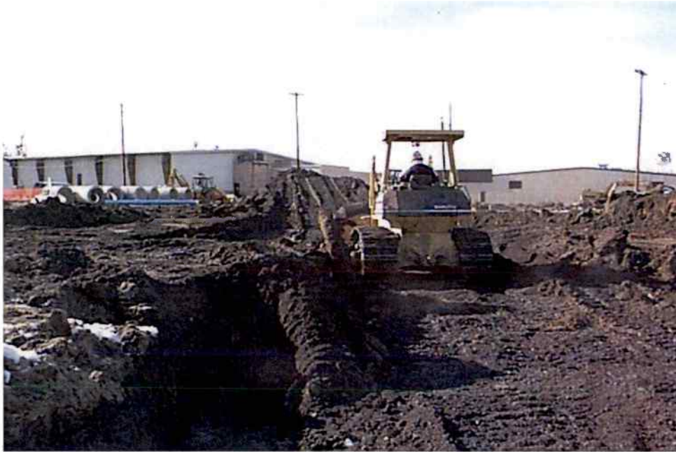
Jan 15, soil excavation from the fuel distribution/railroad track area. The contaminated material was excavated and transported to the ID-27 soil pile staging area.
