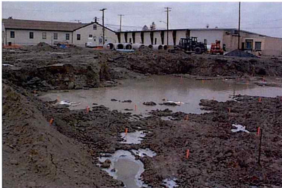
Central excavation area (fuel distribution/railroad track area) sample results show a clean excavation and the area is being backfilled.
